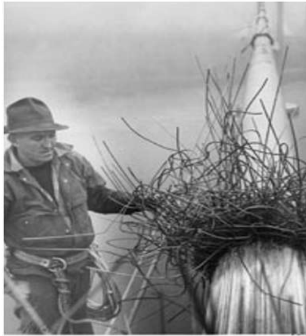
Fig. 10: A bridge inspector examines Damaged cable (Source: WSDOT)
