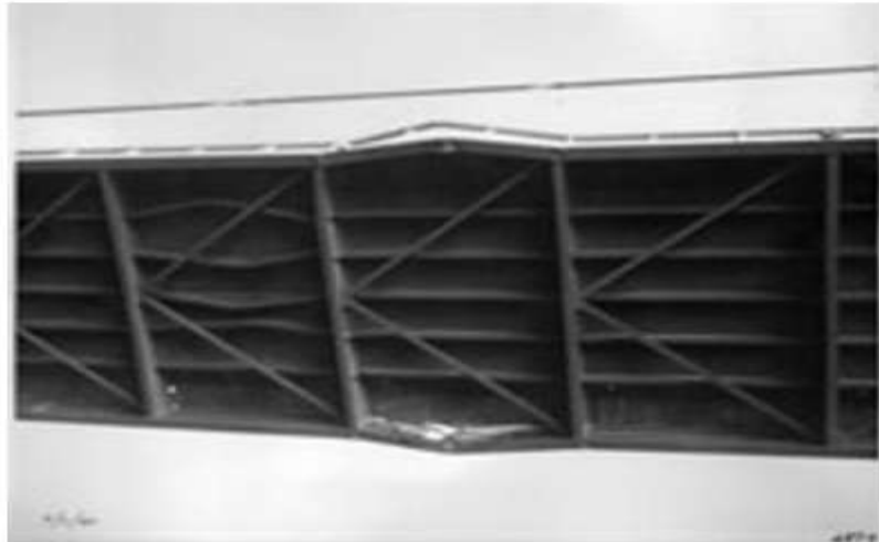
Fig. 12: View from underneath the deck of buckled steel beams. (Source: WSDOT)
